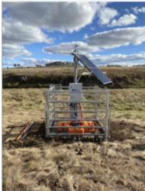
Figure 2 Eco-Detection Ion-Q auto-analyser installed at site GARA2.
